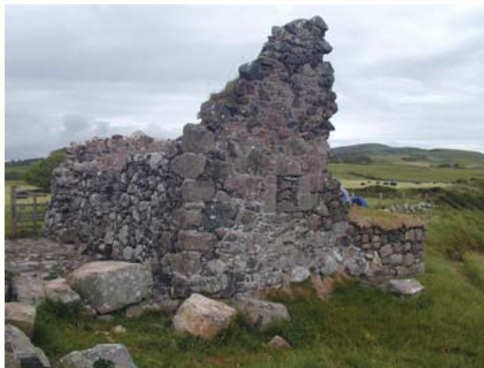
Glenstocken at Gutchers' Isle, Colvend, before and after repair works (© Dumfries and Galloway Council).
